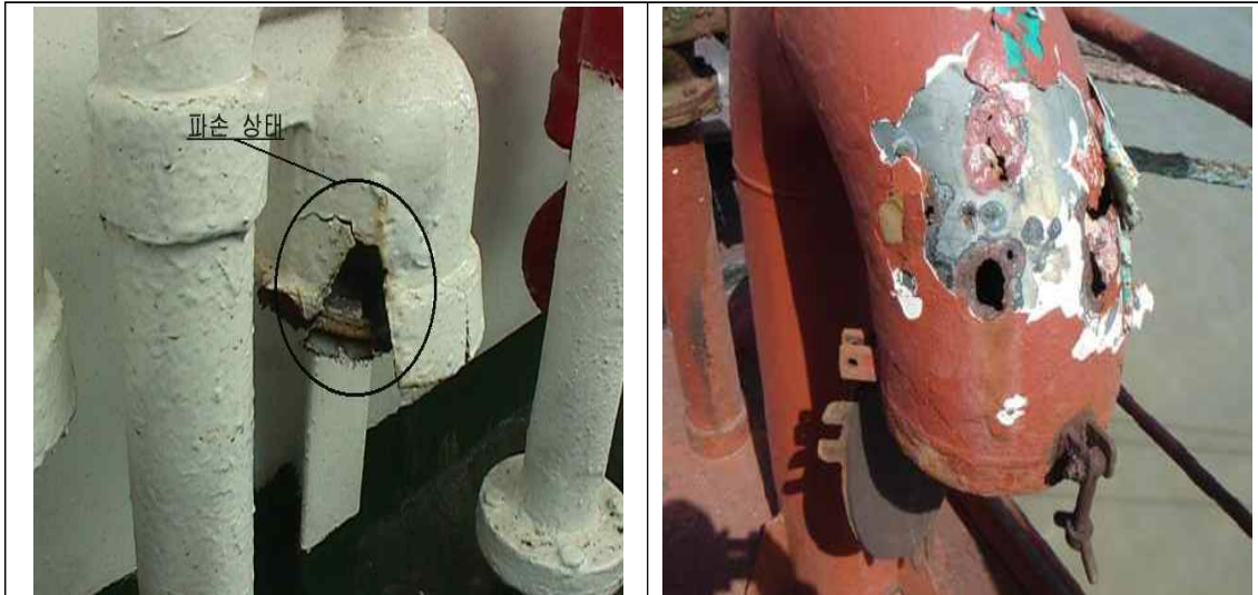
7. External examination of all air pipe heads installed on the exposed decks (Ch 2, 202. 1 (1) (g) of the Rules)
